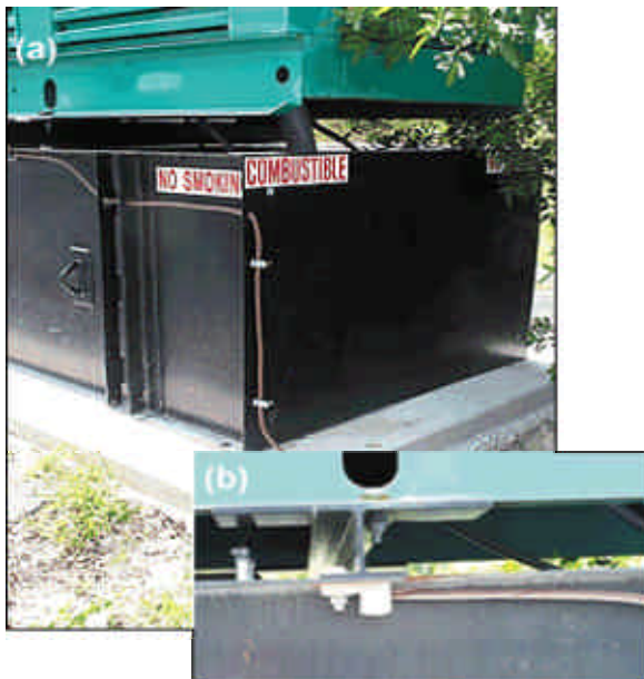
Figure 5a. View of the 4/0 grounding conductor for the 200-kW emergency generator. This conductor is exothermically bonded to the buried grounding electrode system described in the text.
