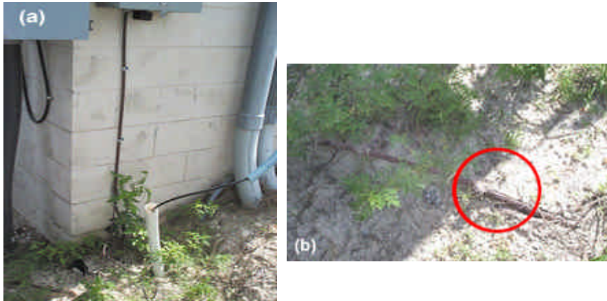
Figure 4a. The main grounding electrode conductor extends from the electrode array to the meter box (vertical cable) and to the service entrance panel seen at upper left. The 4/0 grounding cable leading to the right connects to the air-conditioning equipment subpanel. Exothermic welds ( Figure 4b ) connect the grounding electrode conductor to other outdoor equipment.
