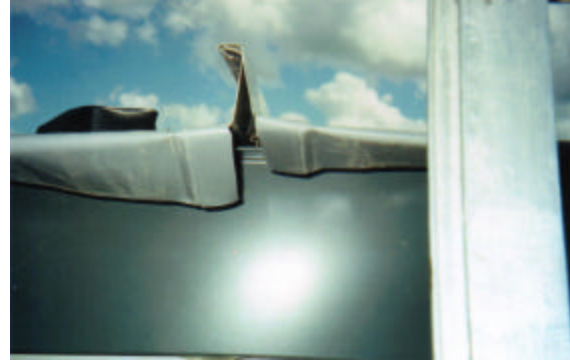
Close up of open, unsealed metal roofing panel edges at eave/gutter and wall connections. This is a waterproofing failure.
