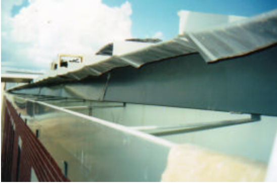
View along eave/gutter line of metal roof. Roof panels are open to water intrusion under the panels and into the building. Building design is zero overhang at eave/gutter and brick wall.
